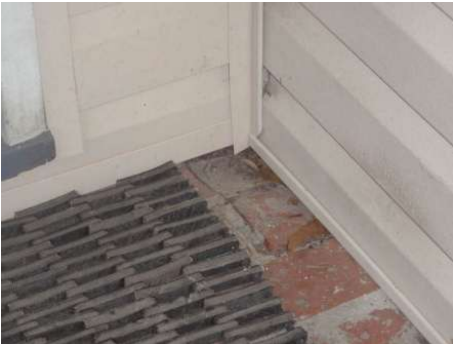
Above: as part of exterior caulking job, this crack in brick, which lets out conditioned air from basement, should be sealed
