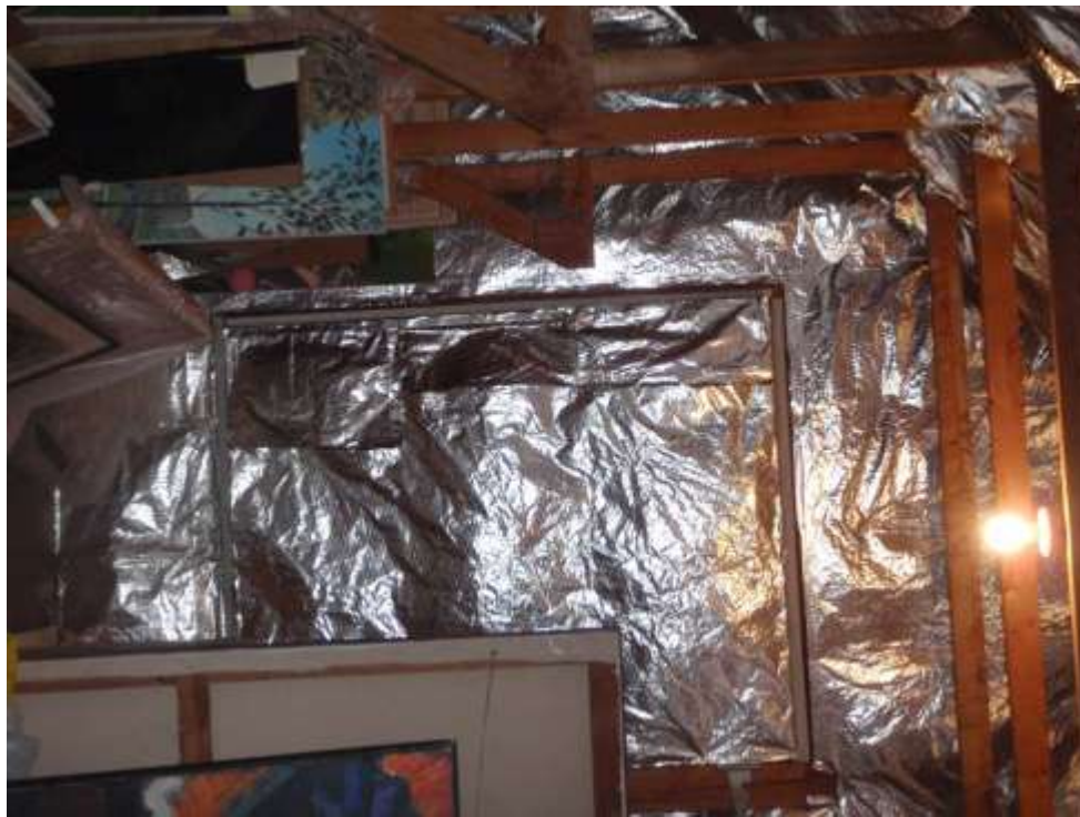
Above and below: cold air entering the perimeter of the attic door above studio; door should be weatherstripped to achieve more constant attic temperatures.
