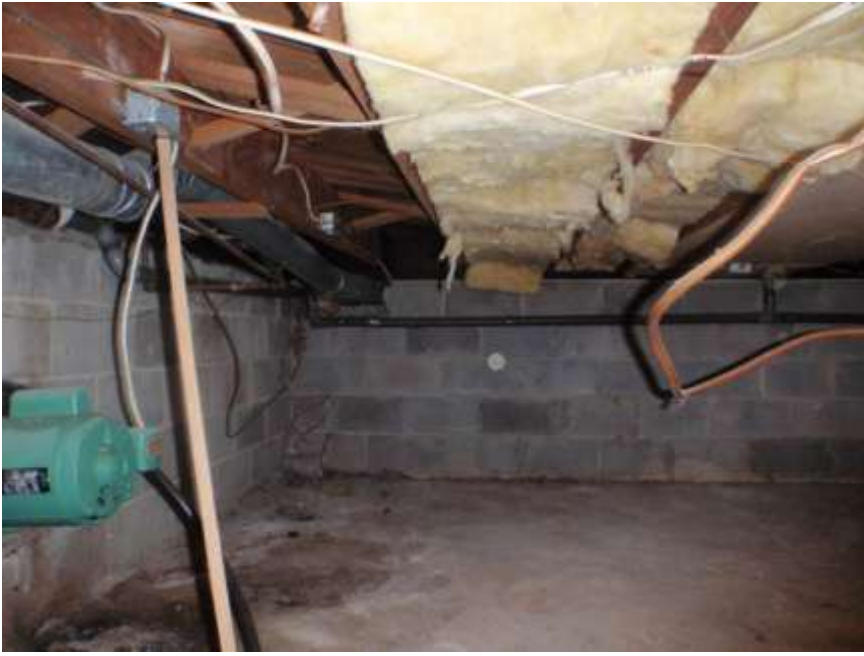
Above: though the crawlspace is well-insulated, it is important to thoroughly air-seal the perimeter of this space
